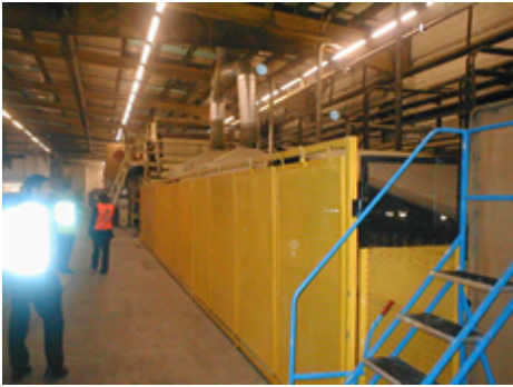
Blanket Press 1 Fence with interlocked gates
